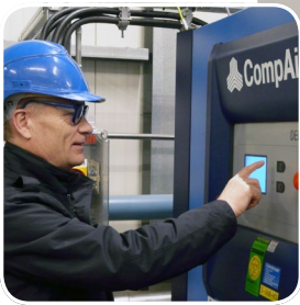
Thorsten Bockelmann, Technical Director of Unimatic GmbH in the compressed air station planned by Unimatic.
