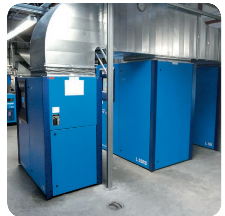
Three highly efficient 50/55 kW compressors, one with speed-regulation, take care of compressed air supply for post processing in the equipment room.
