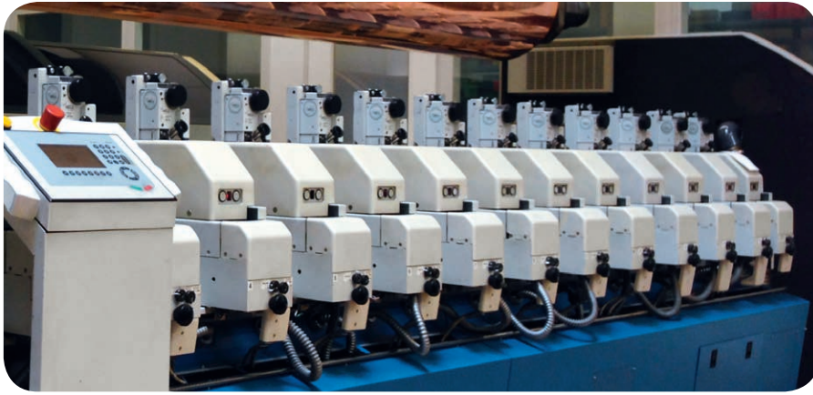
Burda-Druck's Nuremberg site, which was set up in 2001, prints high-quality magazines and catalogues in high numbers. Their compressed air consumption is equally as high: many processes are controlled via pneumatic actuators.
